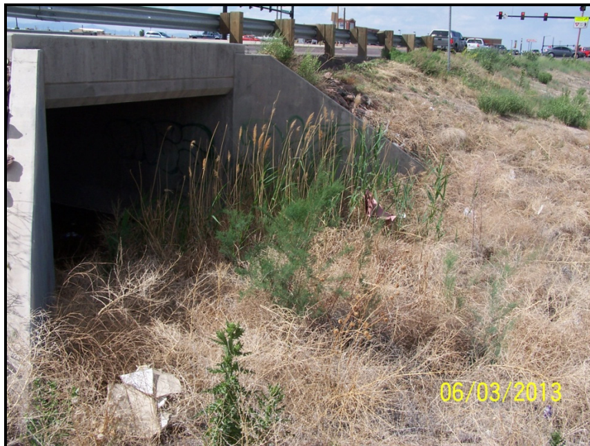
Photo 12 — Looking north next to the concrete box culvert under Purcell Blvd for the tributary to Williams Creek. This drainage is highly channelized and filled with noxious weeds.
