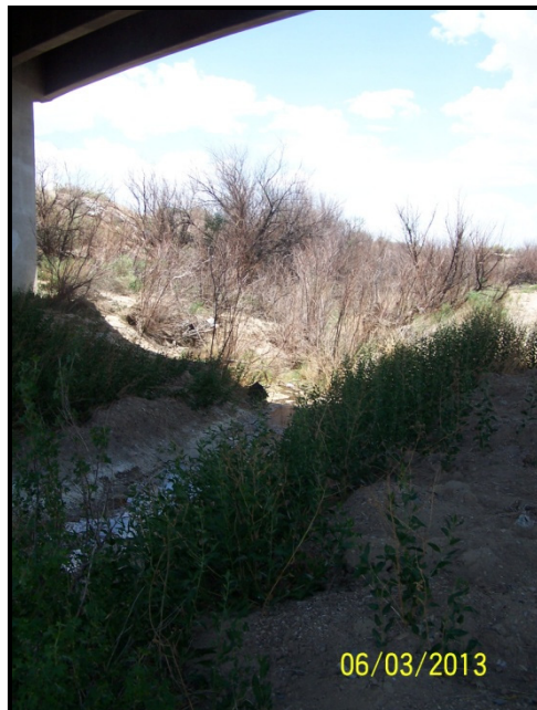
Photo 10 — Looking south from under the eastbound bridge. This channel is very narrow and filled with noxious weeds.
