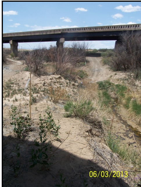
Photo 11 — Looking north from under the eastbound bridge. Pedestrian/off-road vehicle use in the area has eroded and damaged wetlands.
